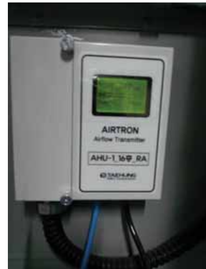
air flow meter
