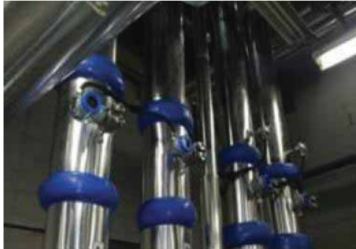
water flow meter
