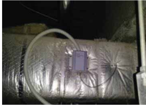
air pressure meter
