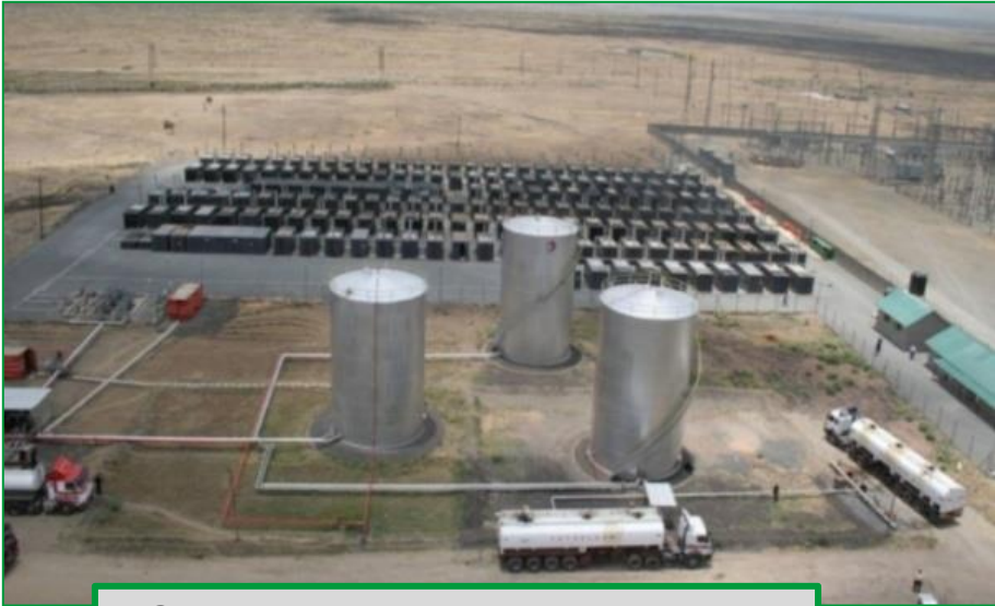
Grid-connected diesel gensets
