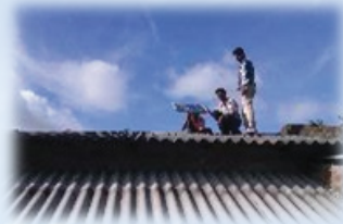
Solar Power Plants
