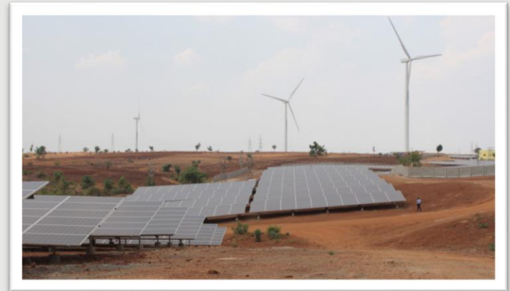
50 MW of the first wind-solar hybrid project owned by Hero Future Energies A 28.8 MW solar PV added to existing 50 MW wind farm to reduce the intermittency of the existing wind farm.
