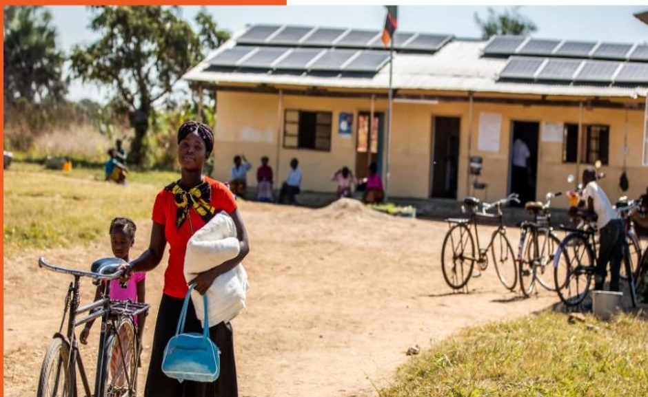
Picture Relevance: Shabasonje, Zambia Health Center. Since the implementation of the solar panels on the roof of the clinic, there is an uninterrupted supply of electricity which ensures that vaccines stay cold and do not spoil
