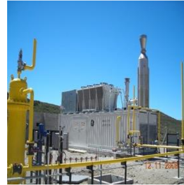
Pipeline gas (Hychico) COD 2008
