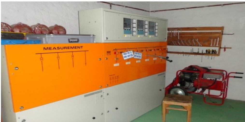
HT Indoor Switchgear Panel
