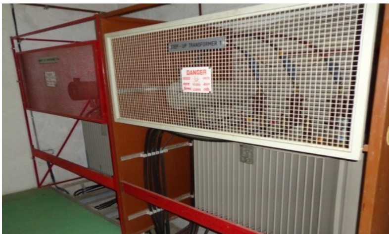
Power Transformer (380V/11000V)
