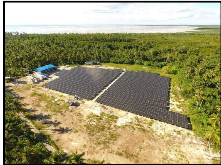
1 Megawatt (MW) Solar PV + Battery Storage System + High Speed Diesel Generator for the Island Municipality of Sitangkai
