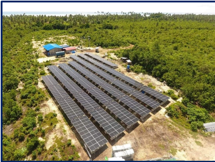
600 Kilowatt (Kw) Solar PV + Battery Energy Storage System for the Island Municipality of Sibuto
