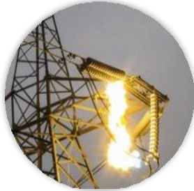
Catastrophic failure due to insulator defects
