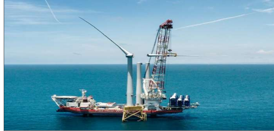
Chang Fang & Xidao wind farm 600MW completed in 2024
