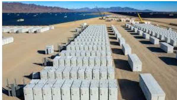
Solar/ BESS Farm
