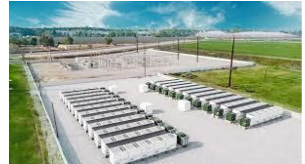
Utility Scale Microgrid
