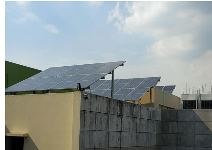
Solar PV with Li-ion battery in Healthcare Centre at Narayanganj, Bangladesh
