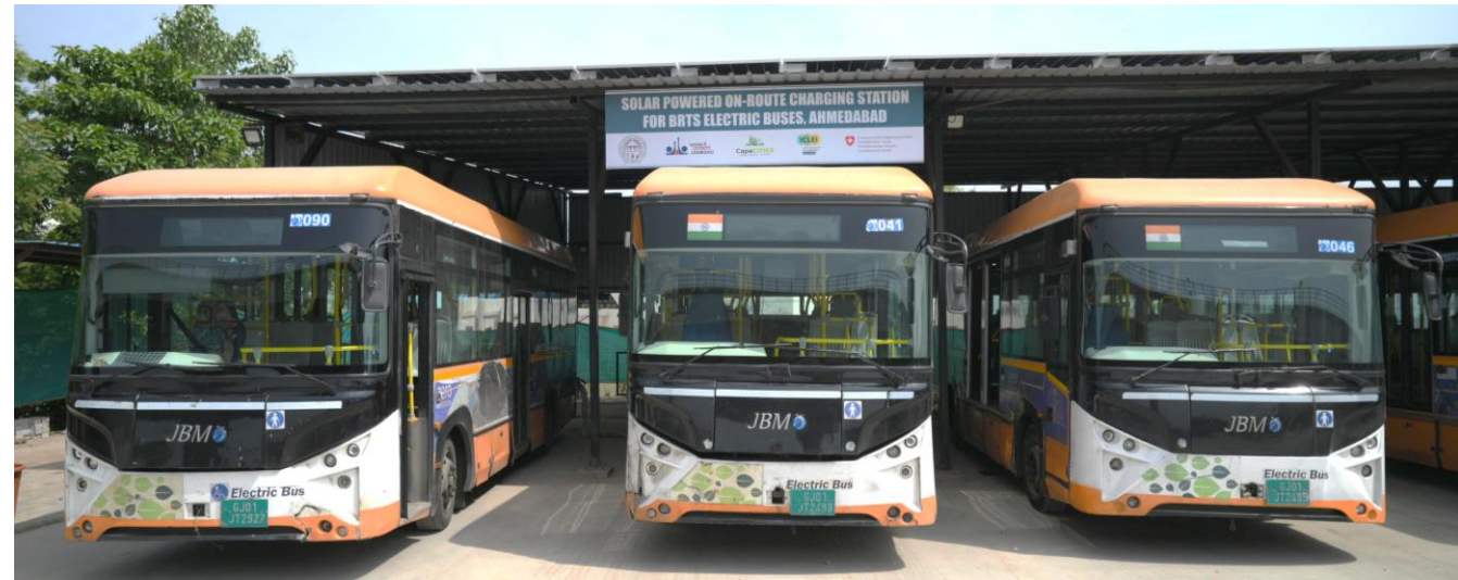
Solar-powered on-route charging facility for public E-buses at Ahmedabad, India
