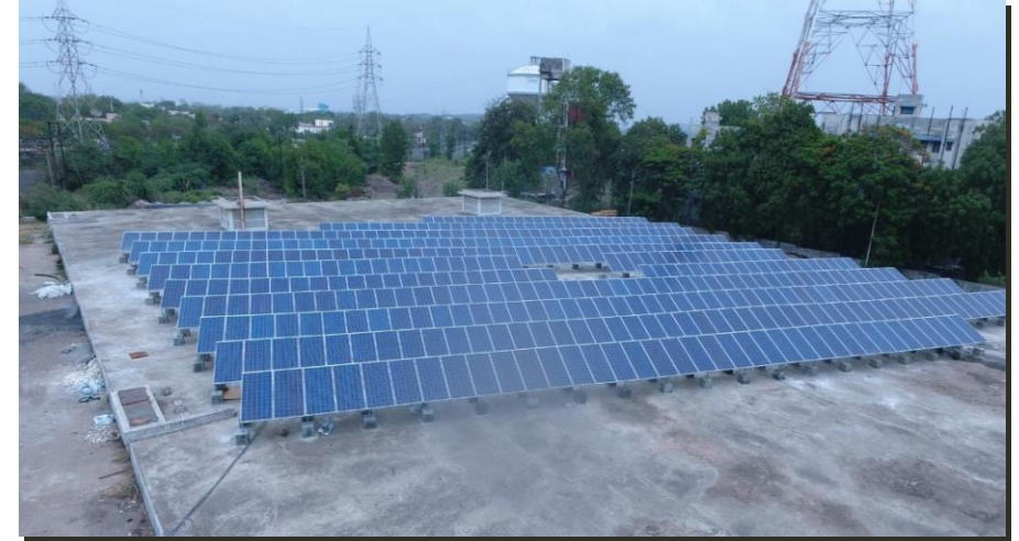
Captive Solar PV at Water Treatment Facility at Rajkot, India
