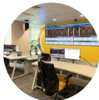
EGAT Demand Response Control Center
