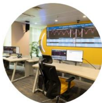
EGAT Demand Response Control Center
